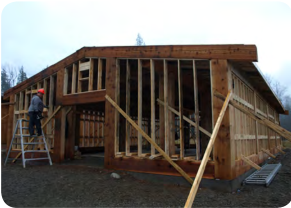
Top photo: Taken October 20th the work on the fourth longhouse steadily progresses. Middle photos: Kitselas Resource employees work on the cedar slats that will become the exterior walls of the new longhouse. Last Photo: Taken November 3rd, excellent progress is being made! The fourth longhouse in the Kitselas Canyon Development is coming along.
